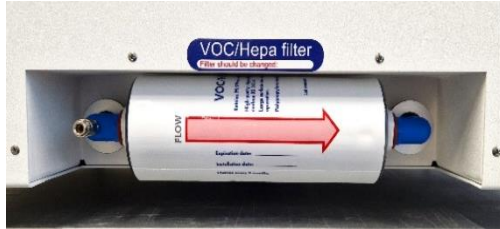
Figure 12.3 Correctly installed VOC/HEPA filter
